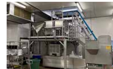
Despite the use of a larger weigher, the system was designed to fit within the existing floorspace and ceiling height.
